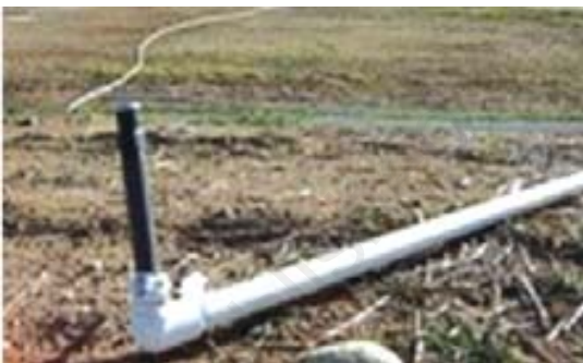
An underground sprinkler system
