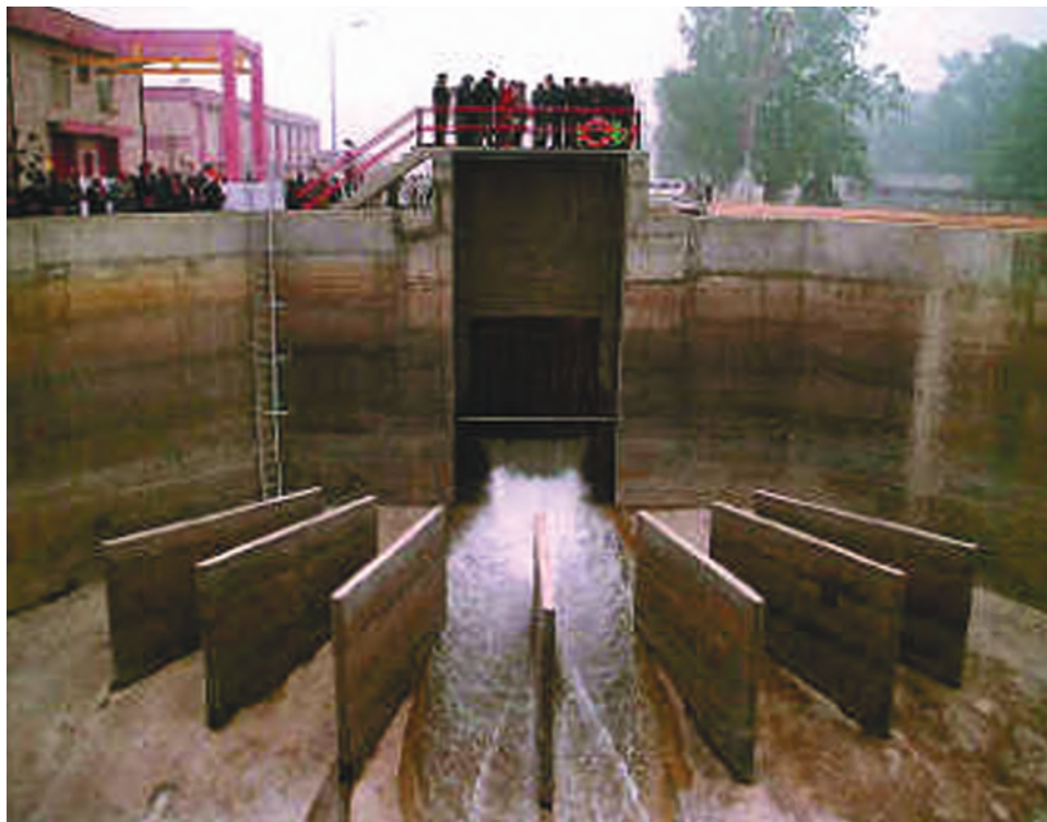
Fig. 18.10 : Water treatment plant
