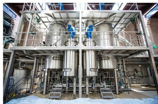
Fig: Fermentation plant
